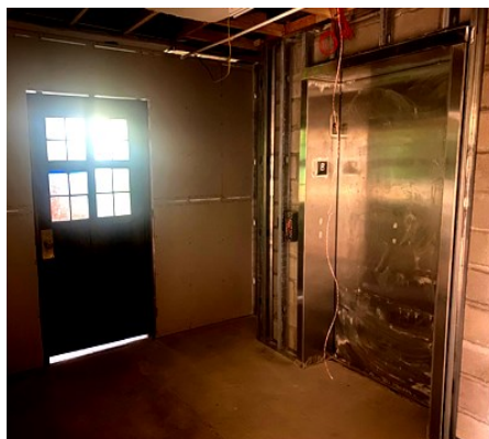
New wall and reuse of Junior Achievement (JA) door at lower level elevator.
