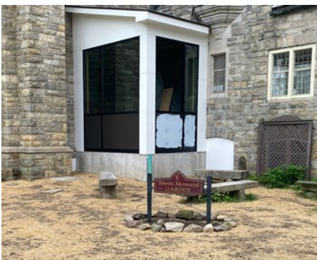
Construction fencing removed and the grass area seeded. The white PVC will be painted gray. Also, the Vestibule for lift at Chapel Narthex.
